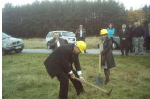
Margarita Petkova, who’s made the environment her priority, turns the first sod of a biomass energy plant, on October 17.
